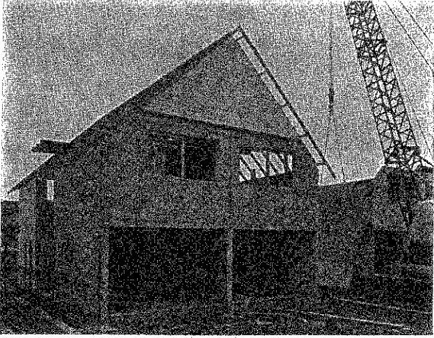
400 dwelling rationalised housing project at Dudley. Precast components form internal skins and all partitions.
